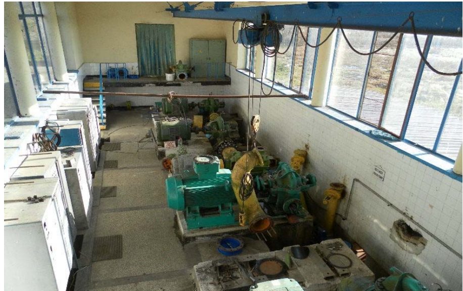
Pumping Station in Dobrich
