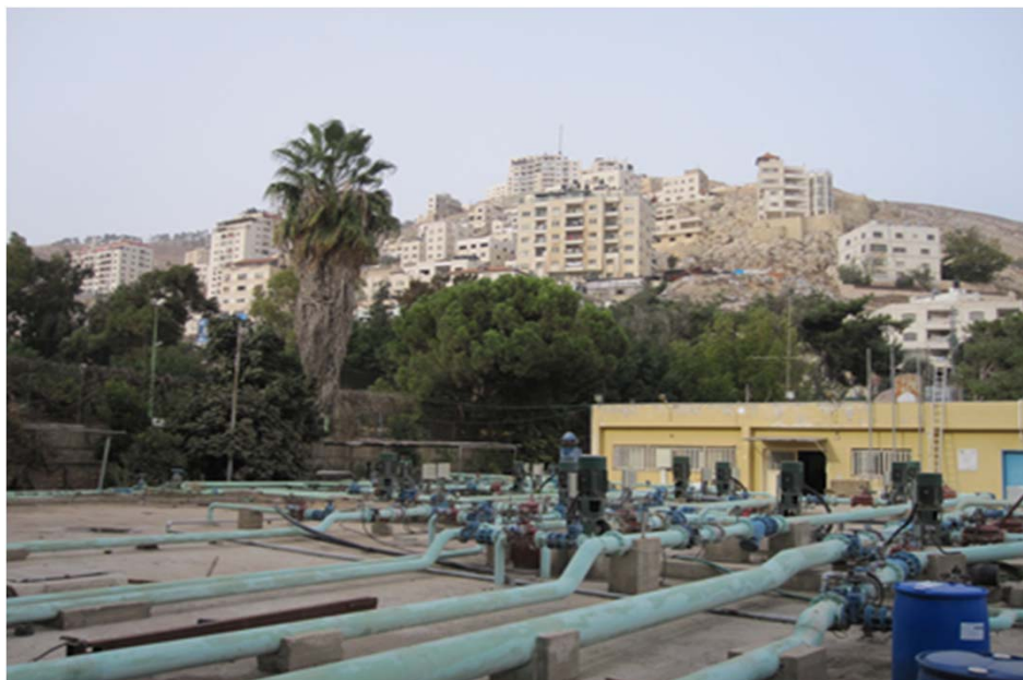
Main Pumping station in Nablus
